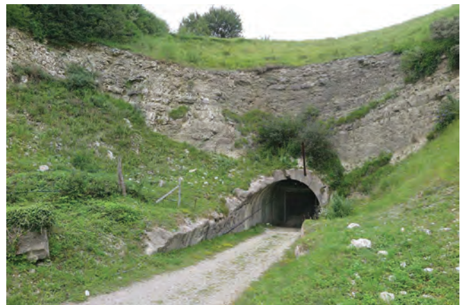
The entrance to the tunnel complex is now thirty metres in from the site of the original portal due to the demolition and subsequent re-excavation. Photo Clive Penfold
